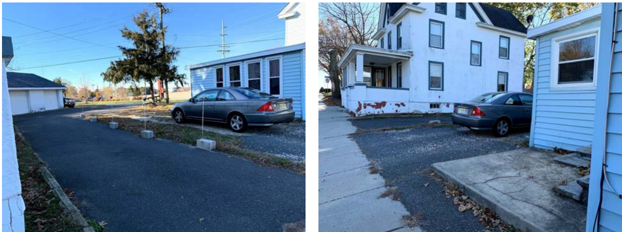
Worn-down and unpaved parking areas (left); cracked entry pads and wear and tear on buildings' facades (right).
