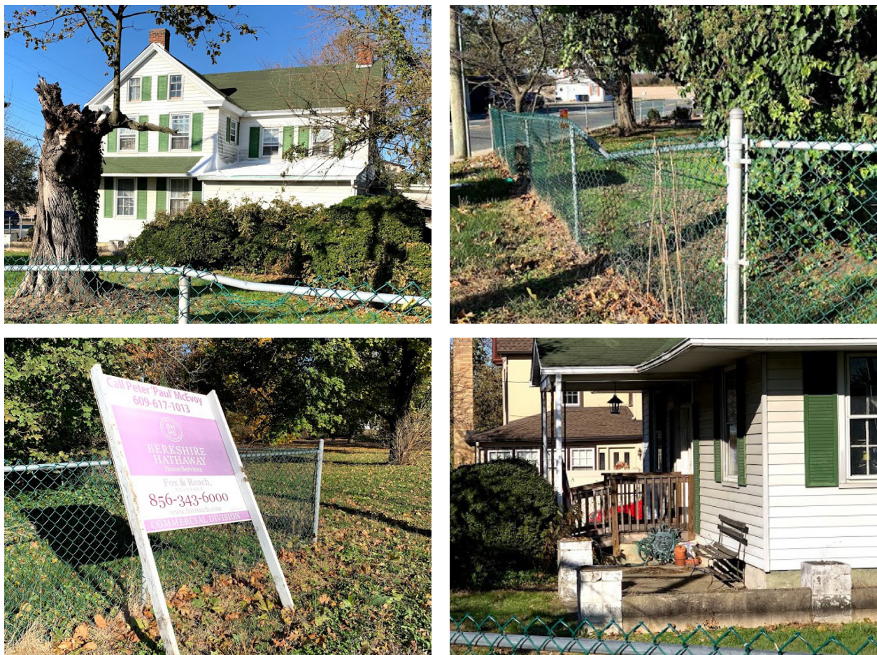
Roof painted white/missing shingles in need of repair (top left); bent fence (top right); "For Sale" sign leaning against fence (bottom left); porch in need of renovation (bottom right).
