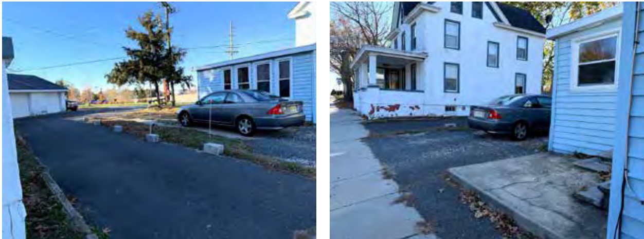
Worn-down and unpaved parking areas (left); cracked entry pads and wear and tear on buildings' facades (right).
