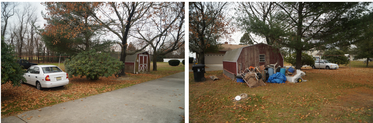
Figure 3. Lot 4: Dilapidated Shed and Debris
